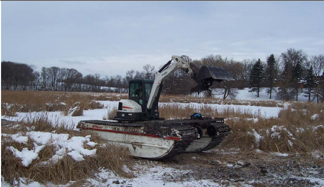
Aquatic vegetation clean out of Lake Independence Outlet Channel, December 2013. Project undertaken with cooperative funding from the cities of Medina and Independence, Three Rivers Park District, and the Pioneer-Sarah Creek Watershed Management Commission.
